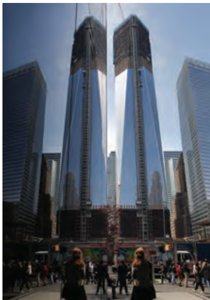
Eye on the Big Apple: Vantone has leased five floors of New York's One World Trade Center, slated to be the tallest building in the US upon completion
